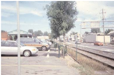
Asphalt removed 15' into the parking lot from the tracks, continuously for 60'. Structural soil placed 30" deep and asphalt reload. Trees in second year of growth after transplanting. Source: http://www.hort.cornell.edu/uhi/outreach/csc/ssoi/sld041.htm
