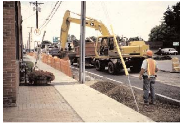
NY State Dept of Transportation installation of CU Structural Soil in Ithaca, NY 1997. Fifty trees of five species planted into continuous trenches.
